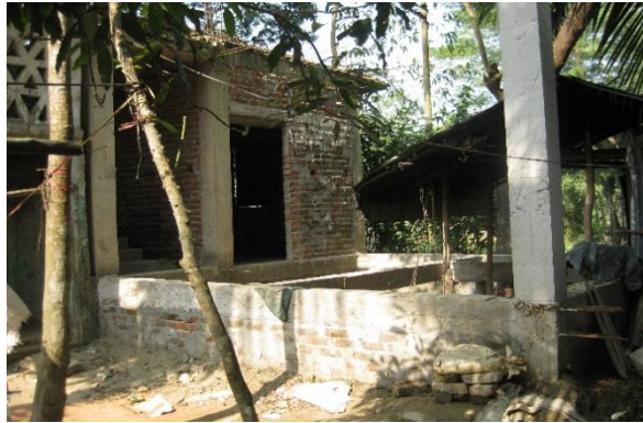
Work is underway to build a house with a loan for business
